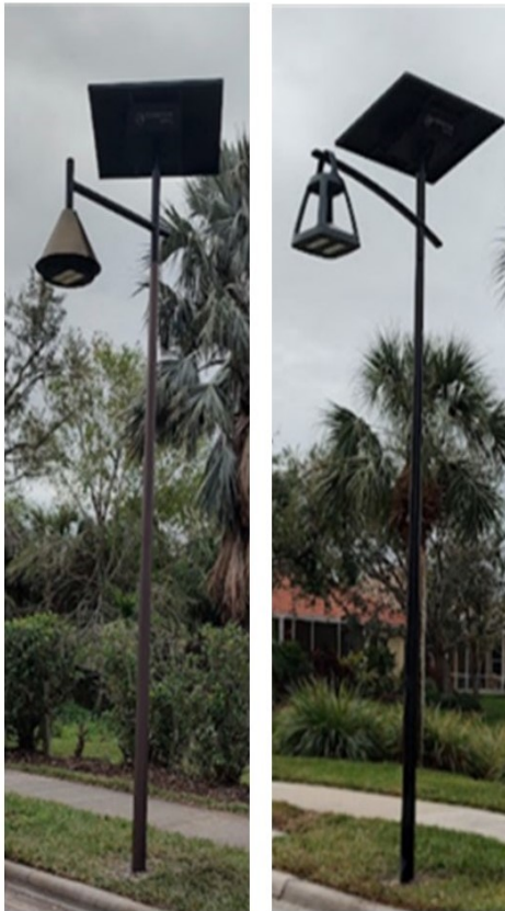
Prototypes just installed mid January, at 100% lumens
